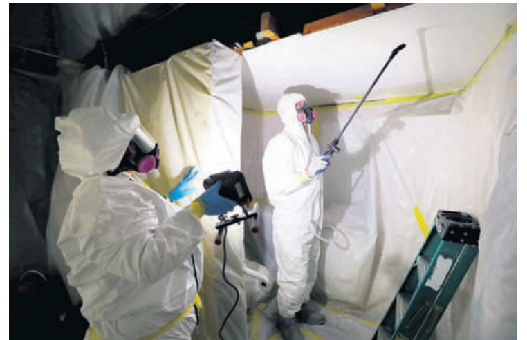
Asbestos Removal Technologies Inc. staff work on asbestos abatement in Howell, Mich., Oct. 18, 2017.
